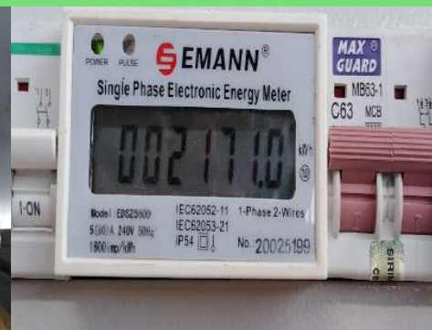
Digital Electric Meter
